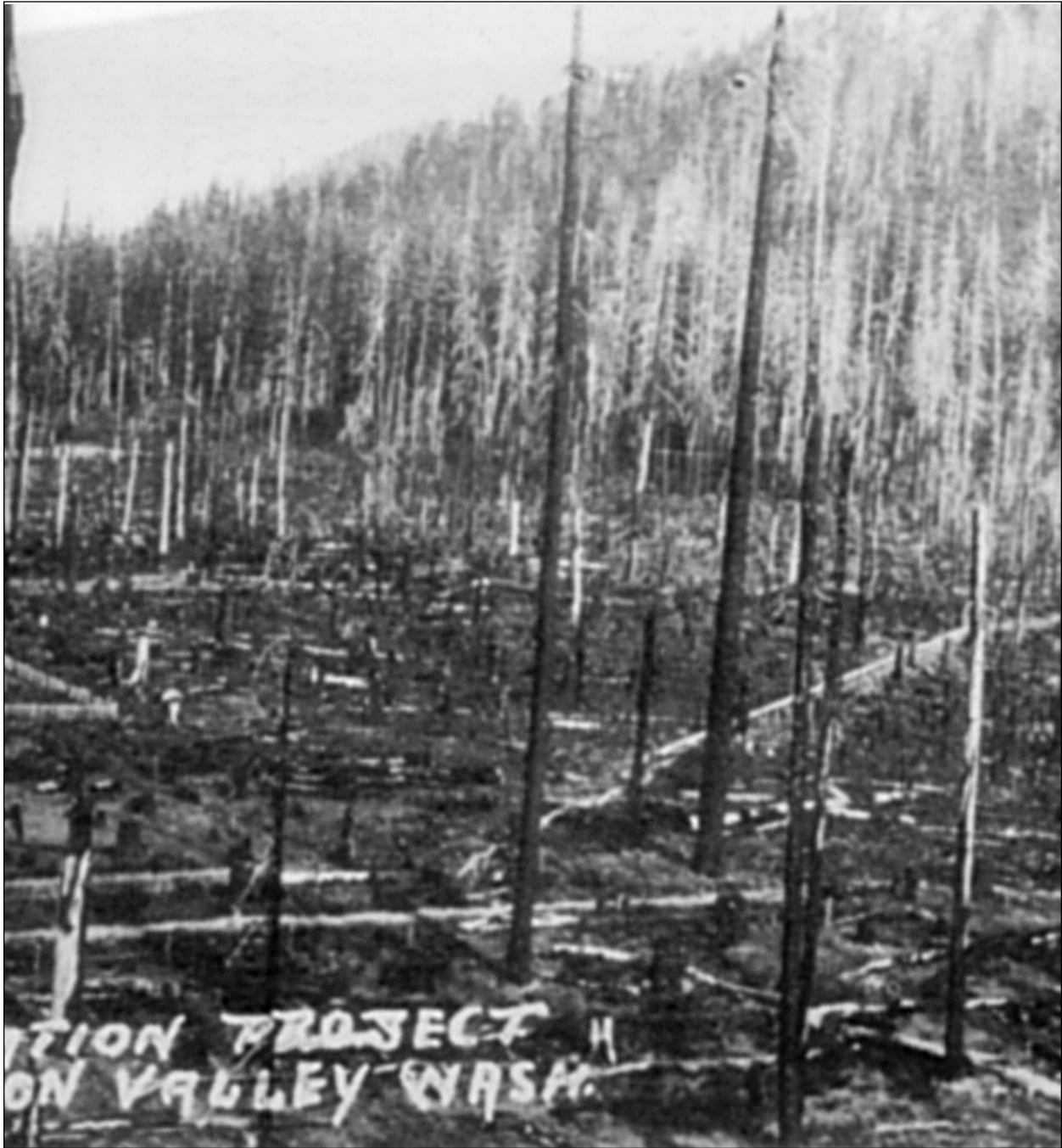
Flume under construction through logged-over land between Panther Creek and Wind River.
