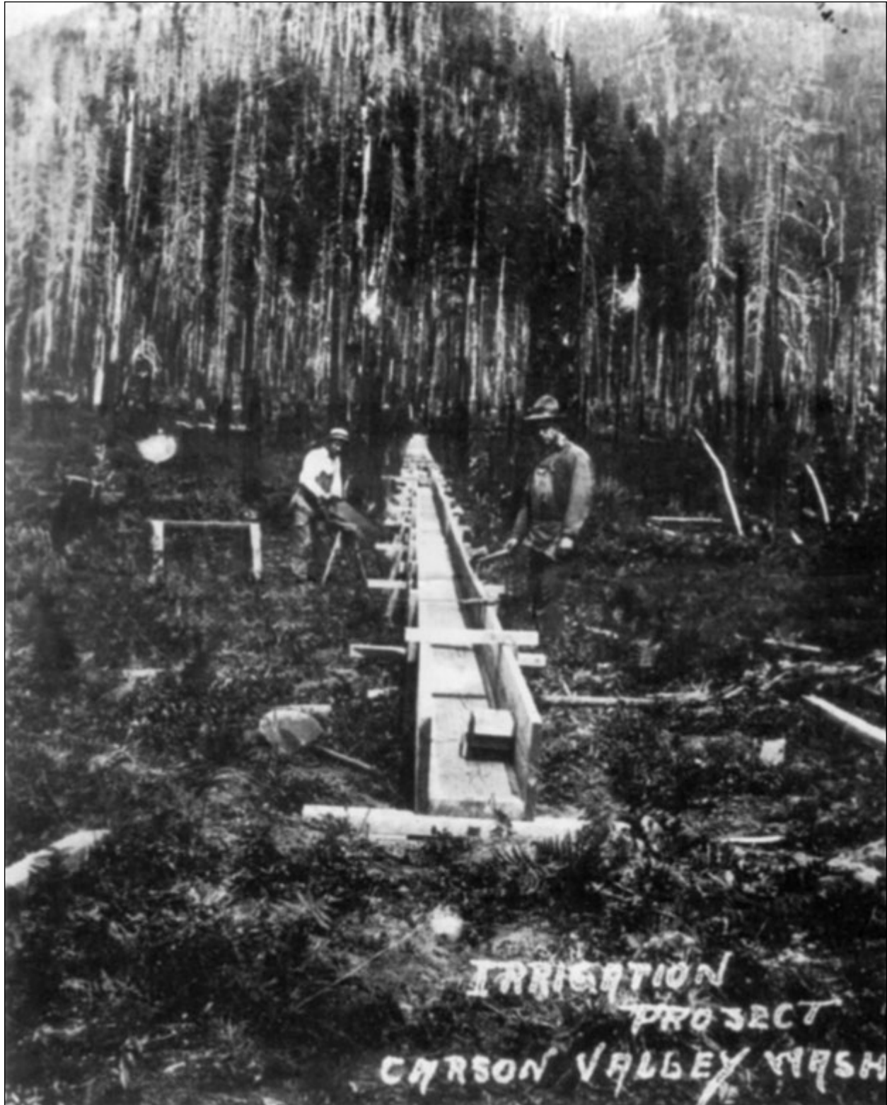
Irrigation project under construction. Flume is built of Douglas fir lumber cut at B. M. Hawley's small steam-powered mill.
