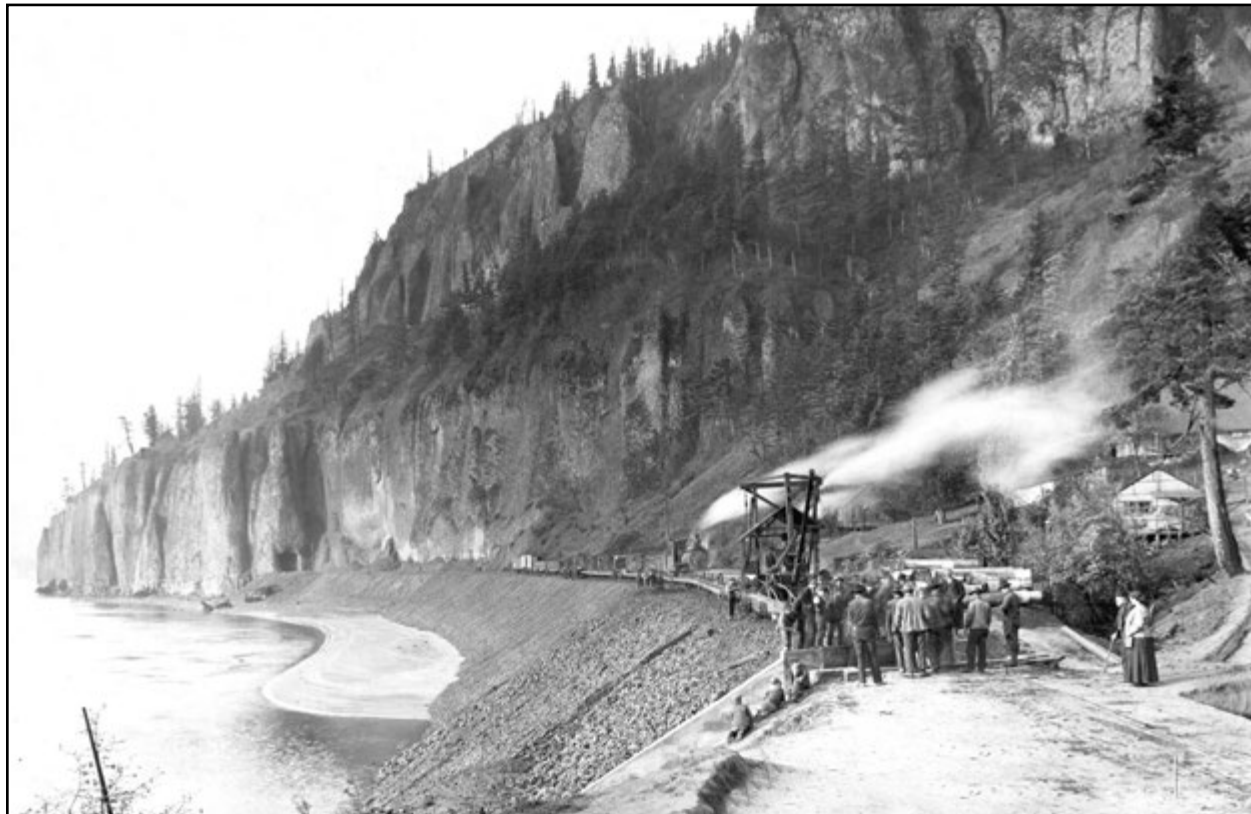
S.P.&S. construction crew and engine "Pioneer" is laying steel at Cape Horn, WA., on Nov. 16, 1907, at 10 a.m. Couple on the right looking on are Mr. and Mrs. John Stevenson, who homesteaded the land at the base of Cape Horn. They are the parents of Emory Stevenson.
